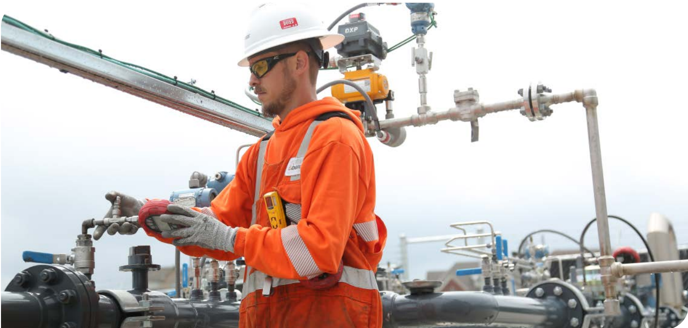
Photo courtesy of Enbridge. Power-to-Gas Facility and hydrogen blending facility in Markham, Ontario
